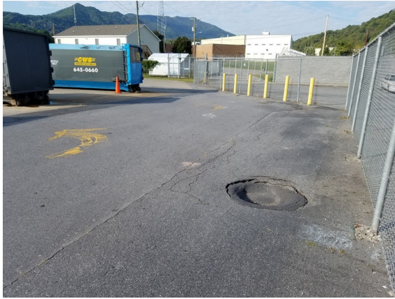
A sunken pothole.
